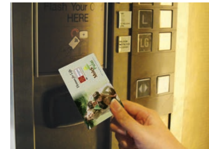
Tier 3: Lift access to specific levels via smart card reader.
