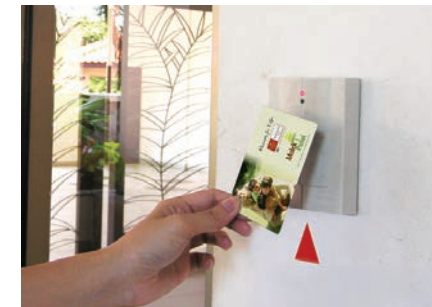
Tier 2: Security Access Card to the lift lobby via car park, and CCTV monitoring system for all entrances, exits and lift lobbies.
