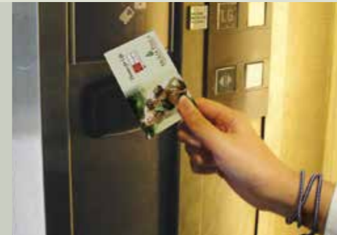
Tier 4: Lift access to specific levels via smart card reader.
