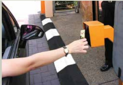
Tier 1: Sensor Access System at the barrier gates of the main entrance and exit.
