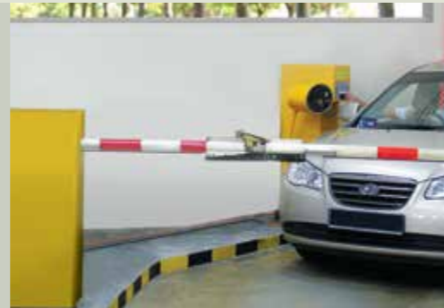
Tier 2: Sensor Access System at the barrier gates of the basement car park entrance.
